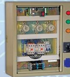
ELPC With Main Power Box
